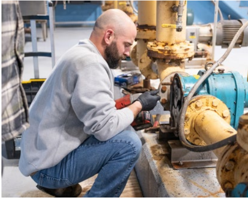
Operator rebuilding Rotary Lobe Pump
