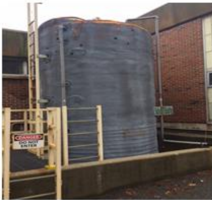
Chlorine and Bisulfite Tanks
